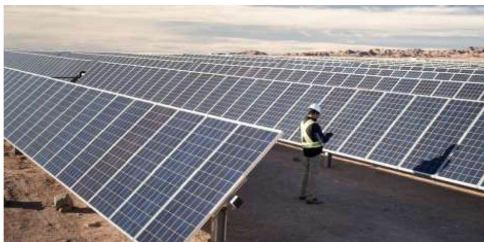
Figure 8: Solar Facility That Supplies Power to Quebrada Blanca Operations
