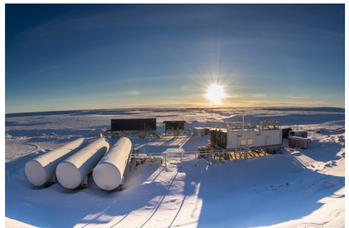
Figure 5. Storage system at Raglan nickel mine, from left to right: hydrogen storage tanks, flywheel and substation, battery system, fuel cells and electrolyser. Source: Natural Resources Canada
