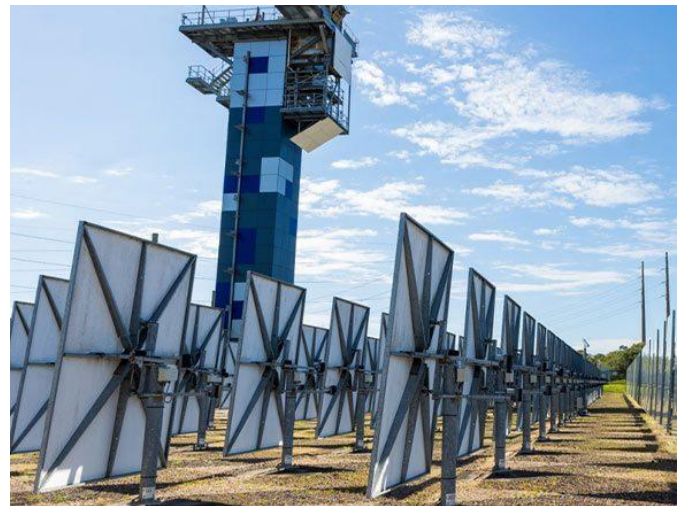
FPR Energy's Newcastle trial installation
